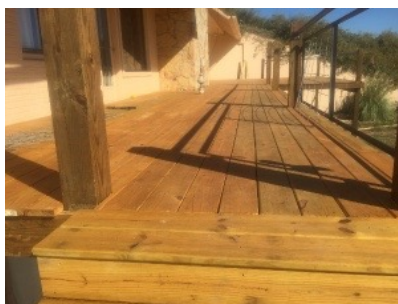
The top portion of the new deck. Larry has also added some soft lighting and hummingbird feeders. Staircases still to be added to access the gazebo on the roof. This house is built into a hill, where we can enjoy the beautiful view from a grassy rooftop.
